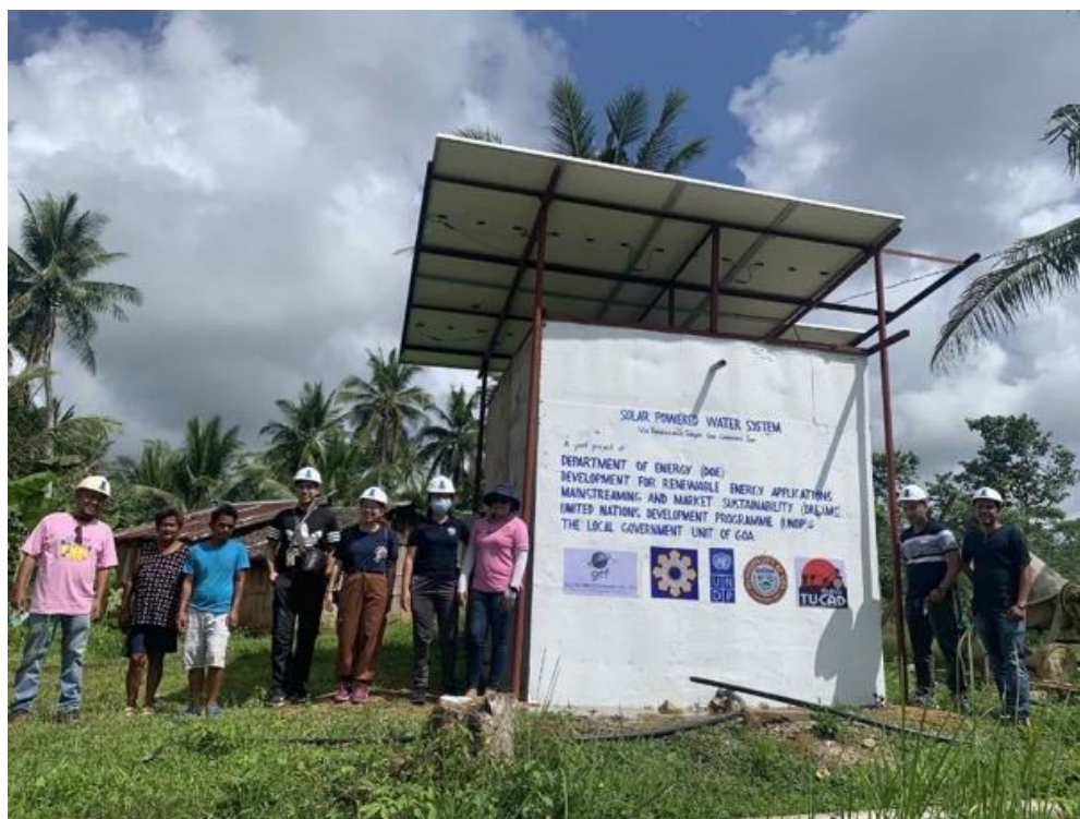
Photo 4. Solar PV Powered Potable Water System in Goa, Camarines Sur Supported by DREAMS
