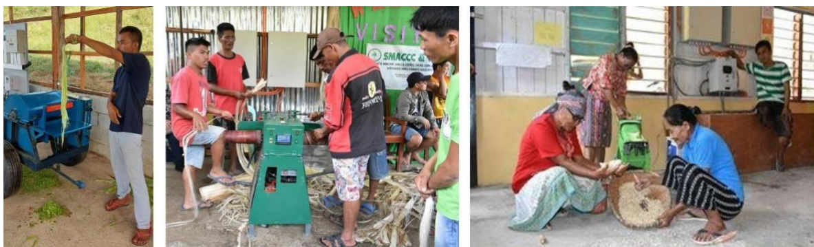
Photo 3. Solar PV-Powered Agricultural Machinery installed by ASEP
