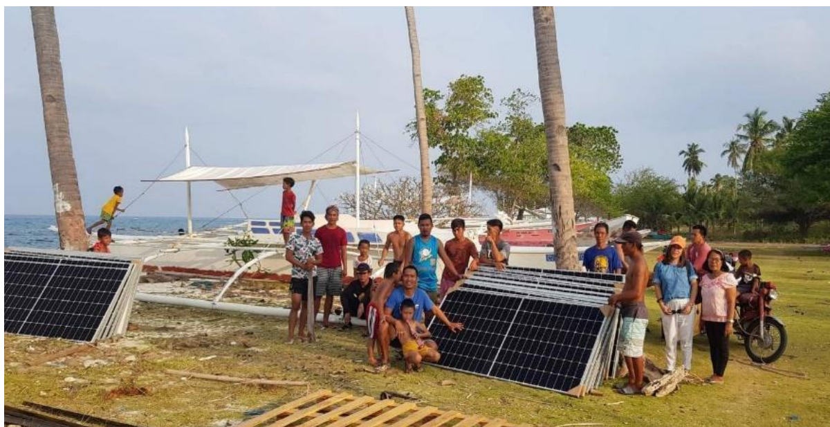
Photo 5. Construction of SF4RE Community Solar PV Project in Off-Grid Pamilacan Island, Baclayon, Bohol
